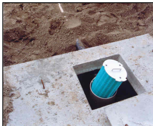
Zabel Effluent Filter (Living by Water Workshop In A Box presentation)
