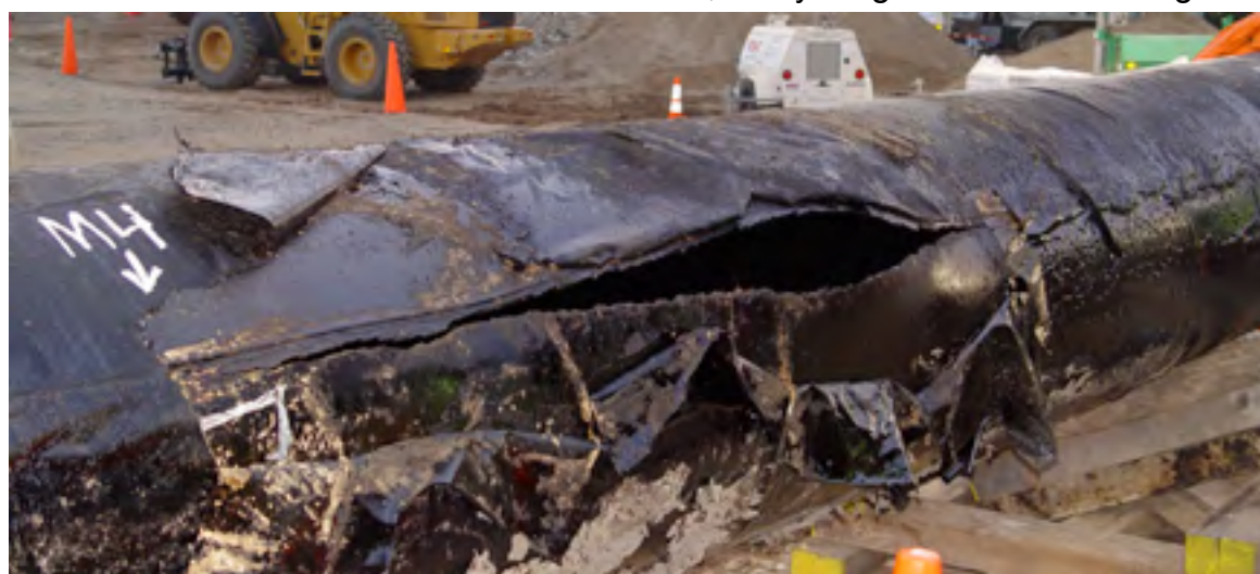
Enbridge’s burst pipeline in Kalamazoo, Michigan
